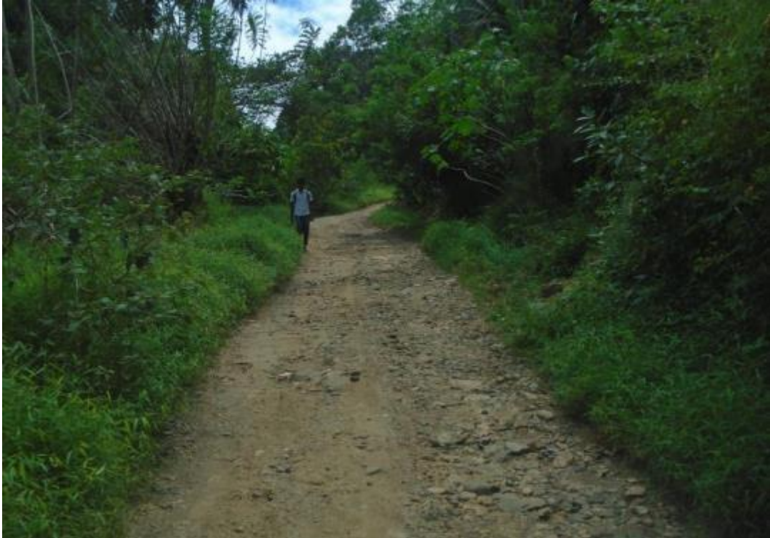
Figure 3: A damaged section of the road
